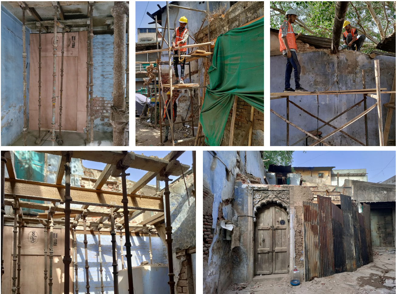
Steps in safeguarding and careful dismantling of the entry structure (photographs by Zeus Pithawalla)
